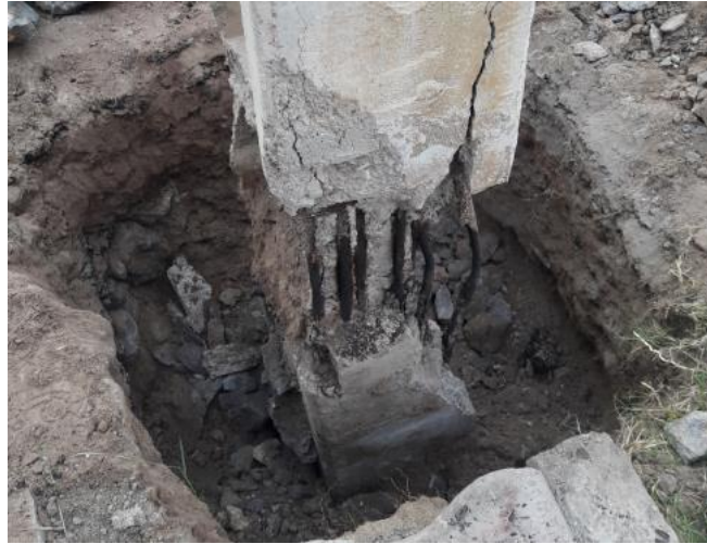
Fig. 1. Anchor damage due to accelerated corrosion
