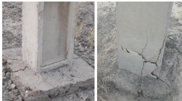
Fig. 2. Severe damage at pole anchors of Armak 'mill lateral (support insulators, concrete backfill, 1997)
