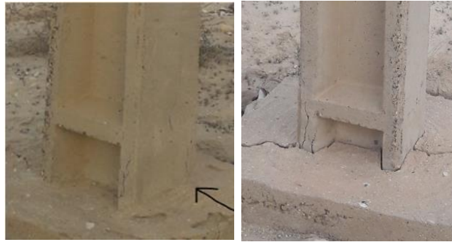
Fig. 3. Moderate damage at pole anchors of Armak main (suspension insulators, concrete backfill, 1991)
